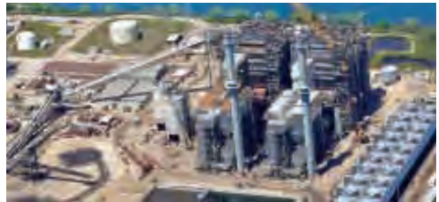
The Oak Grove and Sandow 5 coal-fueled generating units will provide clean, dependable power for Texas consumers.
